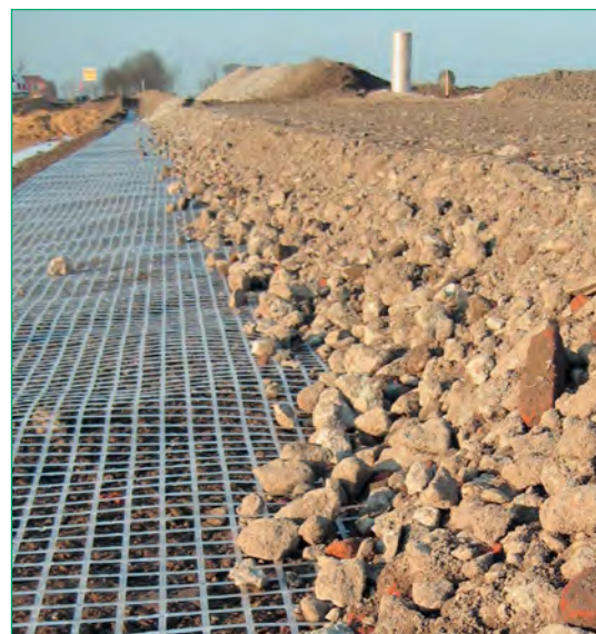
Fig. 19 Crushed base course material over Secugrid® for base stabilisation in access roads
