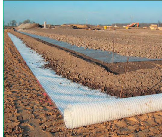
Fig. 8 Base course reinforcement on a very soft subsoil with Combigrid® (bottom) and Secugrid®
